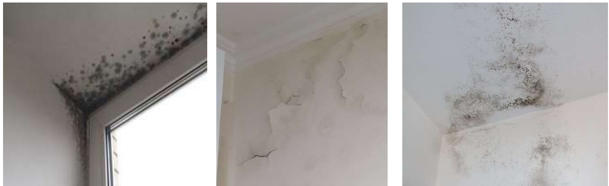
Figure 2. Fungus and deformation of the finish on the inner surface of the outer walls of living rooms
