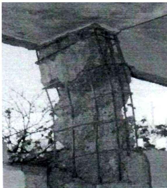
Fig.4 Short Column effect and failure
