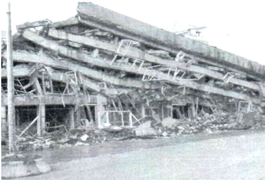
Fig.2 Strong Beam-Weak Column failures
