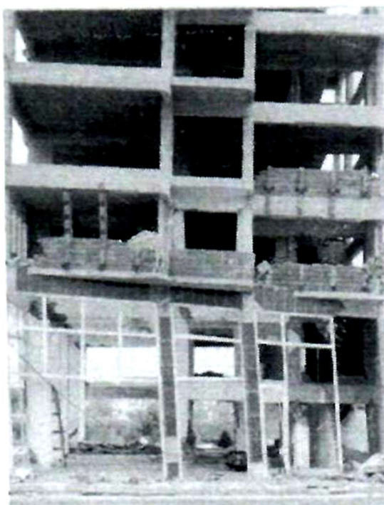
Fig.5 Building with ground floor soft story
