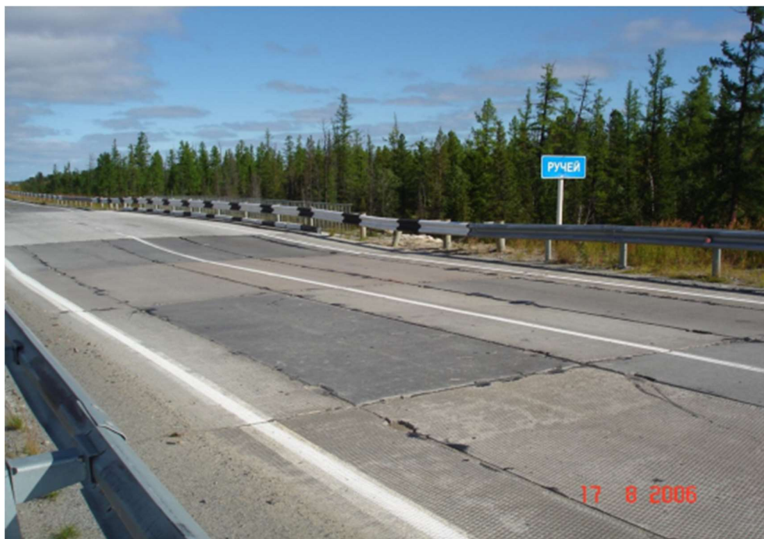
Figure 1 - Deformations of the embankment at the junction with the bridge
