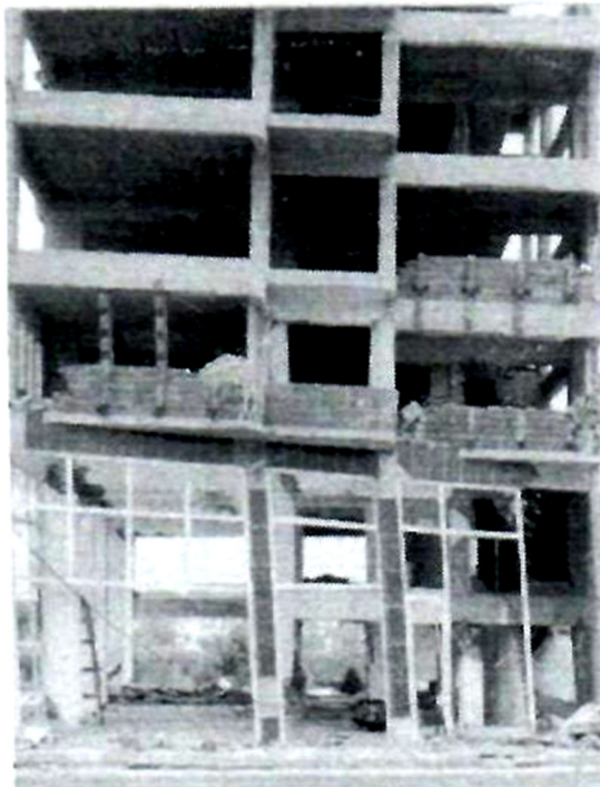
Fig.5 Building with ground floor soft story
